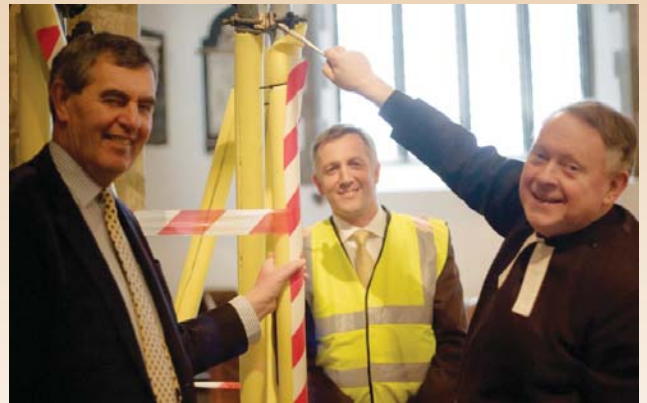
The Dean tightens the last bolt in the scaffolding ready for work to begin on the Cathedral roof. While work is progressing, mid-week morning Services will be held in Chapter House (previously called Cathedral Hall), mid-week evening and Sunday Services will be held in the cathedral itself.
